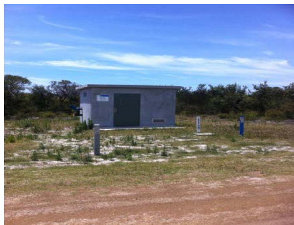
Figure 7: Nabic production bore pump station
