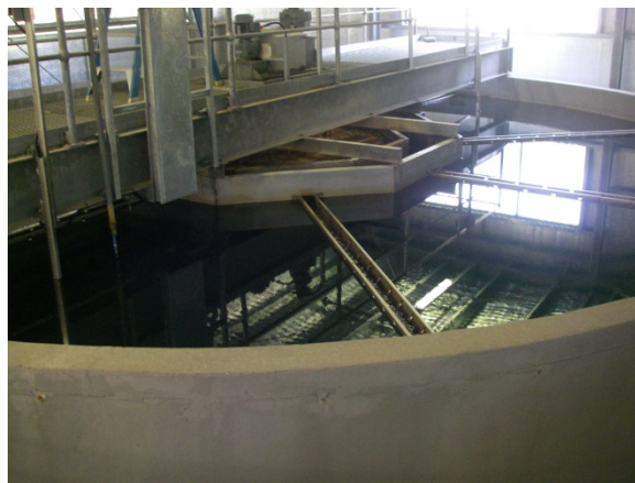
Figure 19: Bulahdelah WTP clarifier
