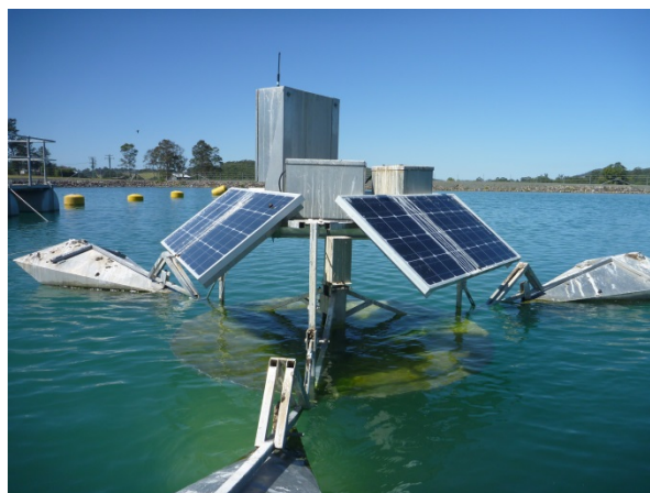
Figure 31: Solar destratifier in off river storage
