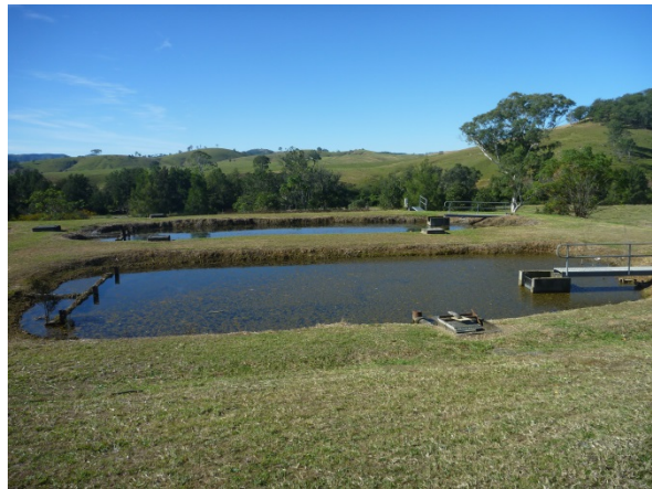
Figure 49: Gloucester WTP sludge lagoons
