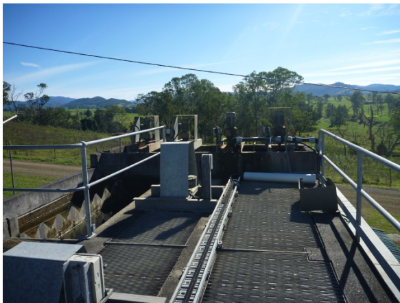
Figure 46: Gloucester WTP mixing chambers
